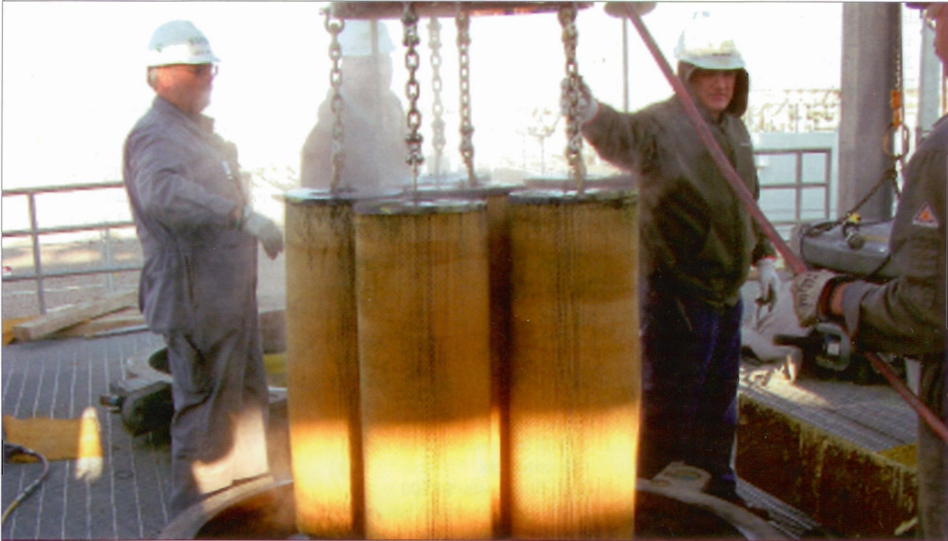
A gas processing plant in Wyoming using this new cartridge filter technology.
