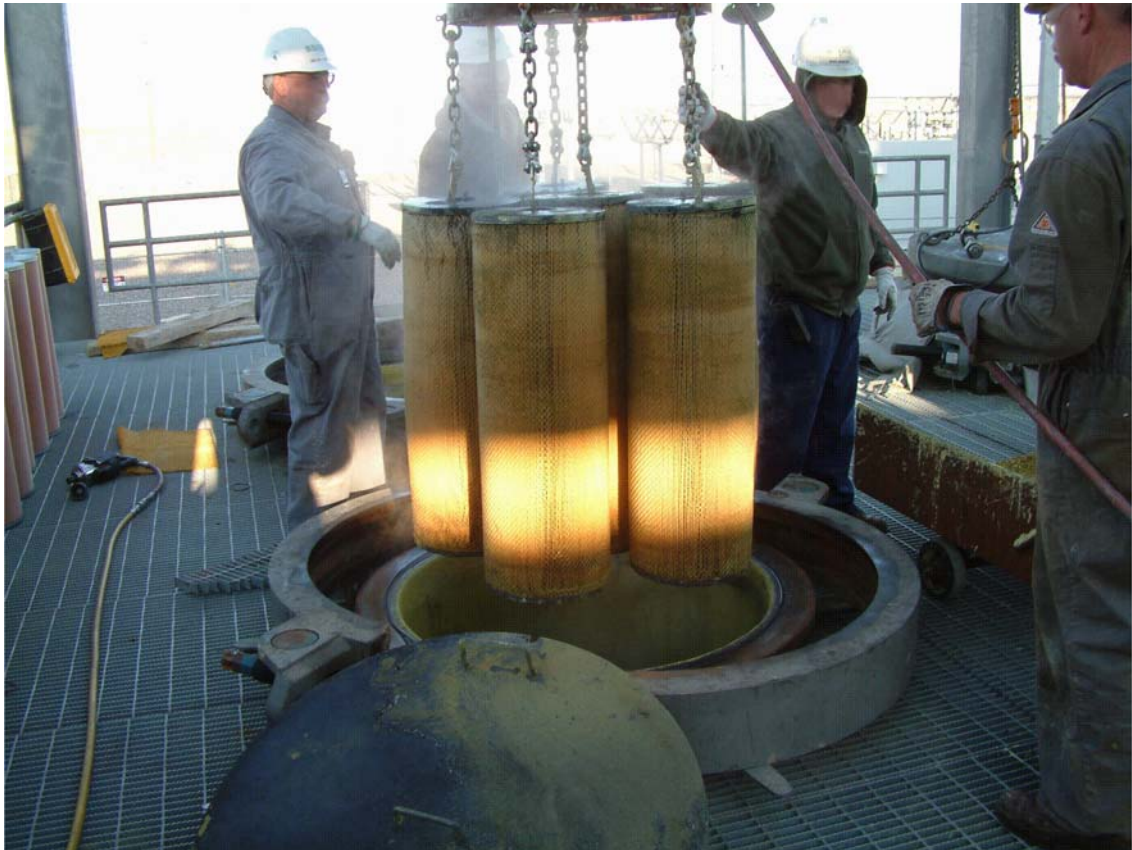
GAS PROCESSING PLANT IN WYOMING (12.75" FILTER)
