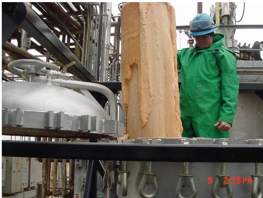
WEST TEXAS CHEMICAL PLANT (12.75" FILTER)
